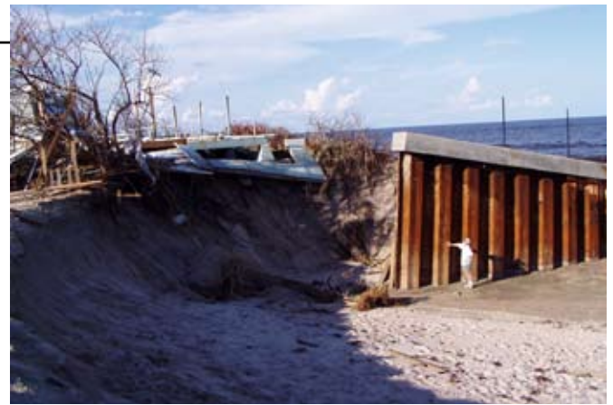
STC's Gary Appelson standing in front of an exposed sea wall in Brevard County after a hurricane
